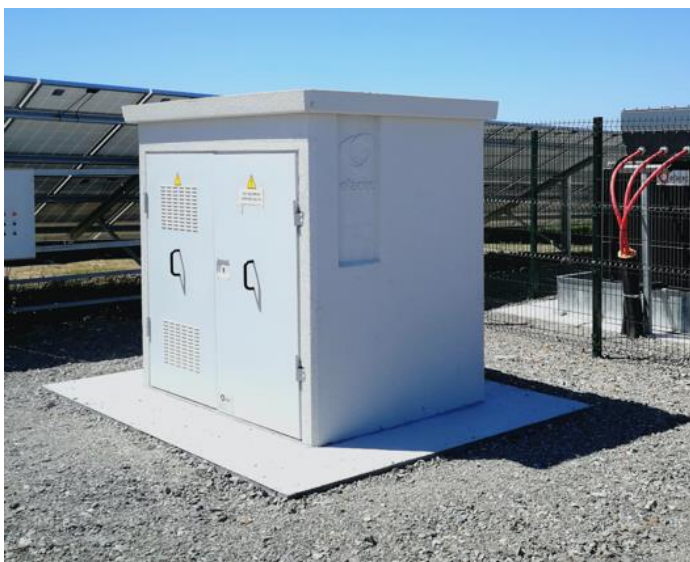
Photo 2-12: Typical cabin indoor switchgear used in the 'outdoor solution' (as per Supporting Infrastructure Option A)
