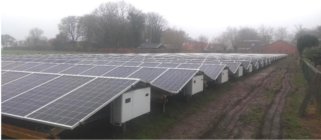
Photo 2-4: Solar panels with east-west facing configuration ( image reproduced courtesy of Huawei )
