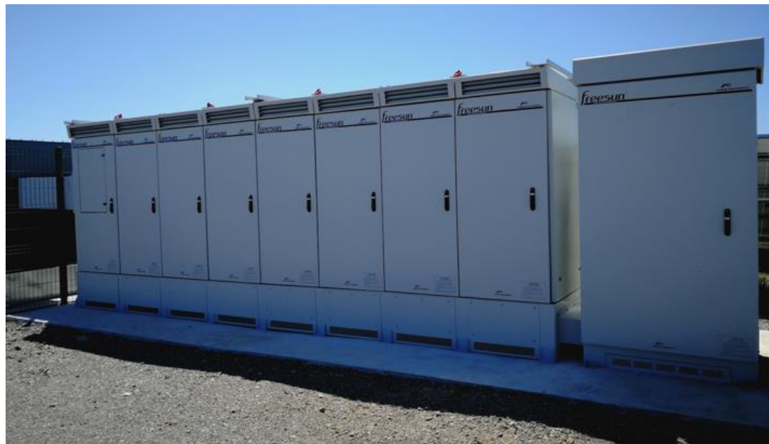
Photo 2-9: Typical outdoor centralised inverter (as per Supporting Infrastructure Option A)
