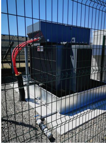
Photo 2-10: Typical outdoor transformer
