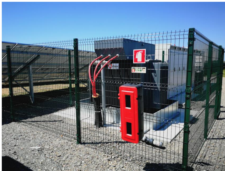
Photo 2-15: Typical transformer compound fencing
