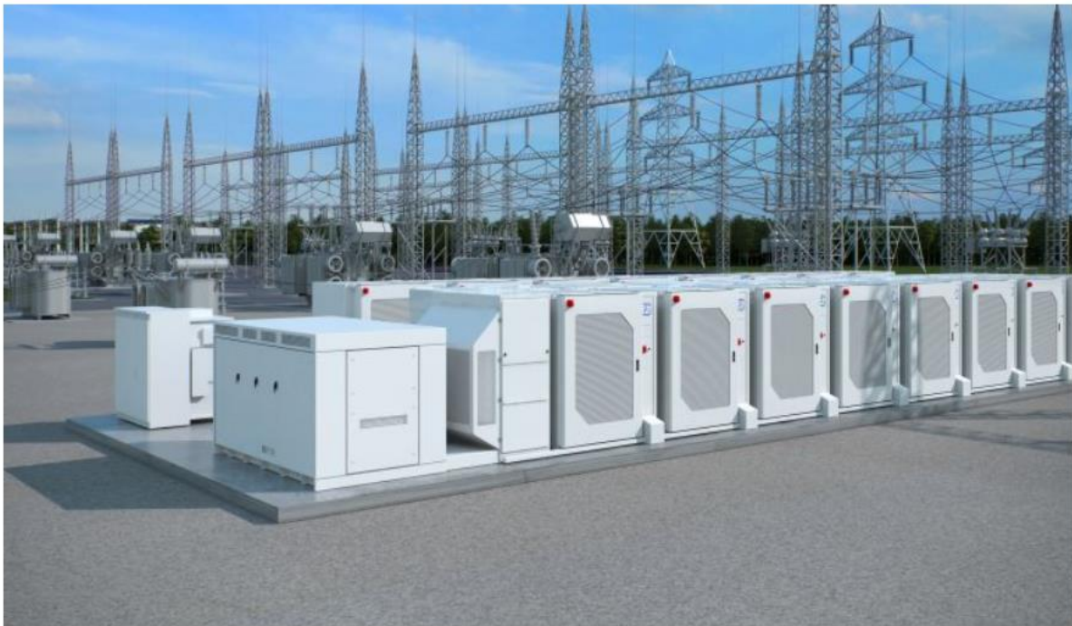
Photo 2-13: Example Battery Storage facility
